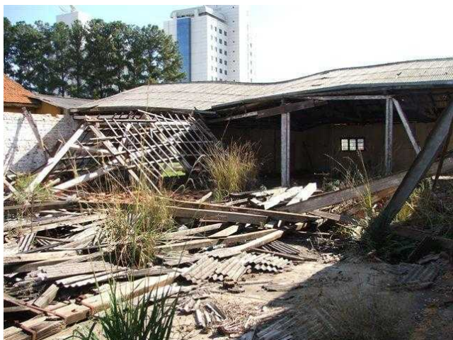
Decommissioning of the Wagner Wall Division plant in Ponta Grossa, Paraná. Photo: Fernanda Giannasi.
